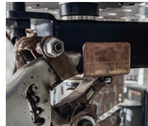
Built-in grounding point
